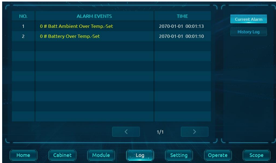
Figure 5-16 Log (Current Alarm)
